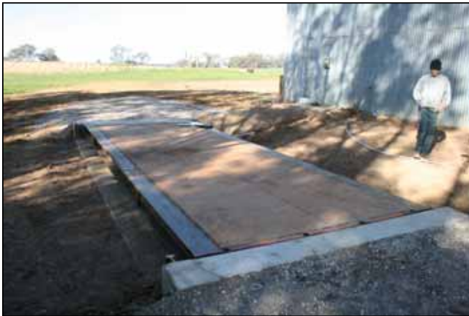
David Spence's Weighbridge in place and ready to go
