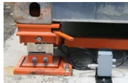
Close-up of the one of the 12t loadcells
